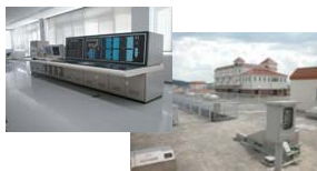
Electric instrumentation systems for water and sewerage
