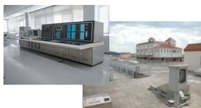
Electric instrumentation systems for water and sewerage
