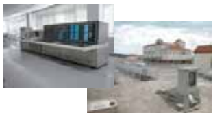
Electric instrumentation systems for water and sewerage
