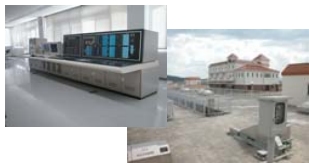
Electric instrumentation systems for water and sewerage
