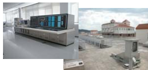
Electric instrumentation systems for water and sewerage
