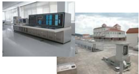
Electric instrumentation systems for water and sewerage
