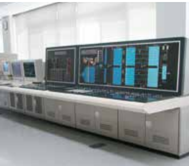
Sewage activity monitoring room
