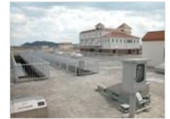
Electrical instrumentation systems for water and sewerage
