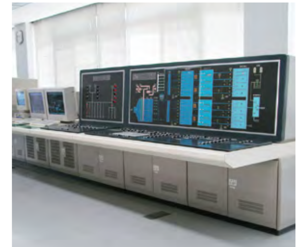
Sewage activity monitoring room
