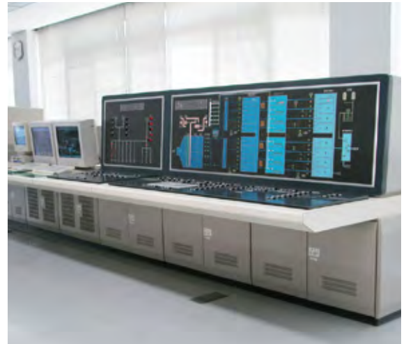
Sewage activity monitoring room
