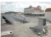
Electrical instrumentation systems for water and sewerage
